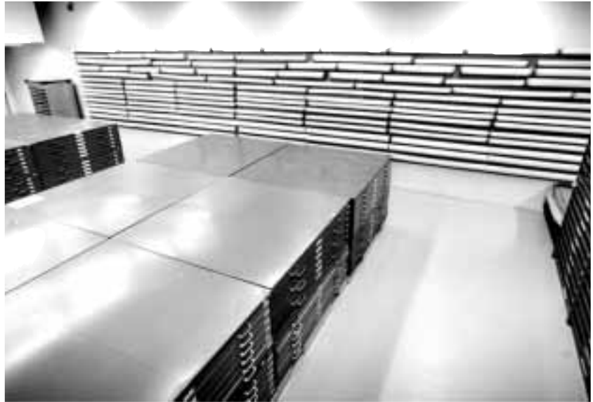
Storage of rolled documents in tubes suspended from the wall. National Archives of Canada, Ottawa, photo Denis Gagnon. ©
