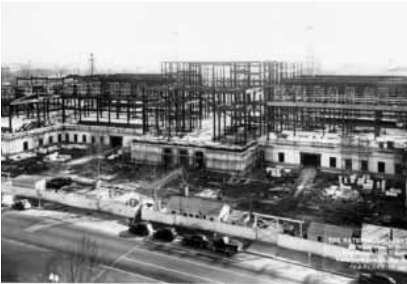
Photograph. Construction view of the National Gallery of Art, Washington, D.C. showing the steel superstructure, 1939.
